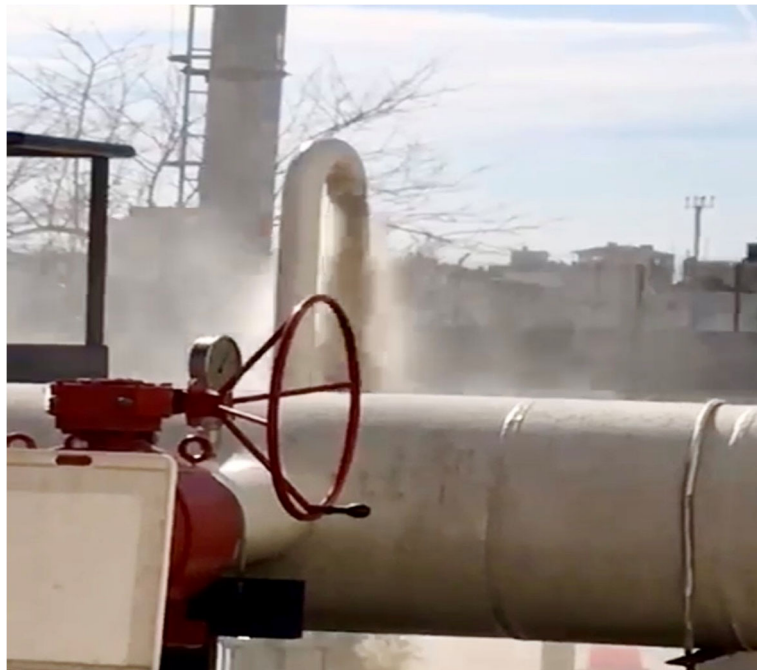
Figure 1. Condensed Liquid Blow-Out from City Gate Station at 55-70 Bar.
